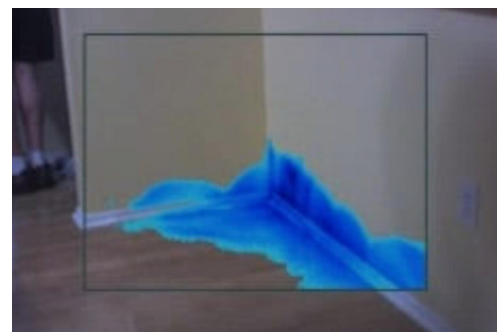
Thermal Leak Detection
